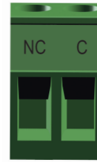
Relay output in the control box
