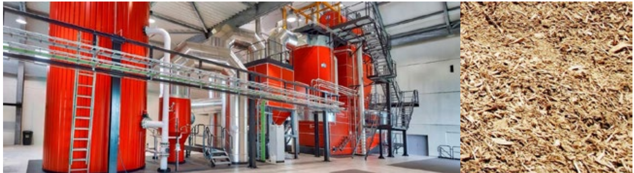
Main boiler – Kathrine and close-up of wooden chips
